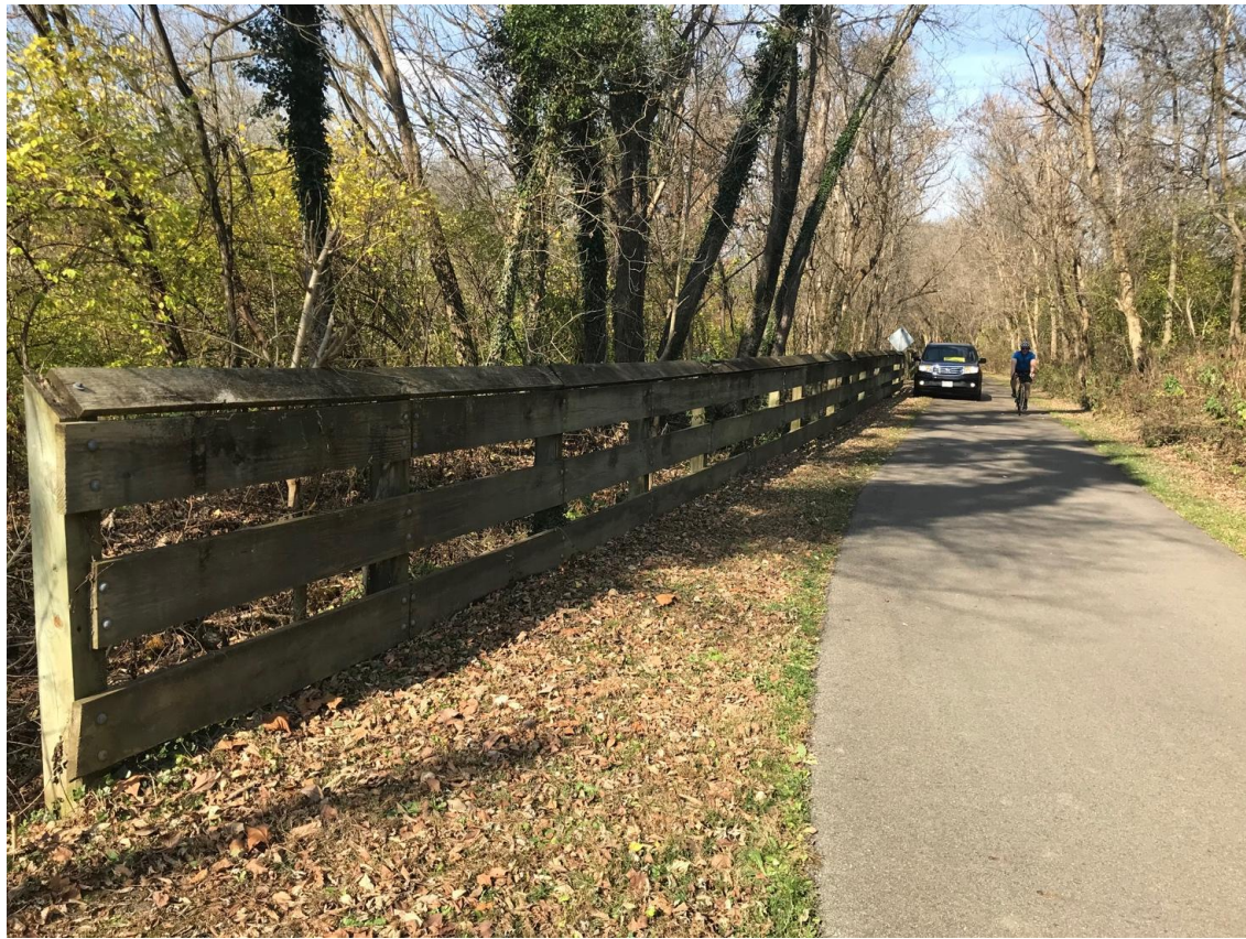
Mile Marker 25: Horizontal boards are a miscalculation from a project 10 years ago. Some of these boards may be used for needed repairs in other areas.
